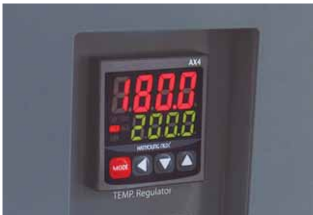
Individual over temperature limiter
